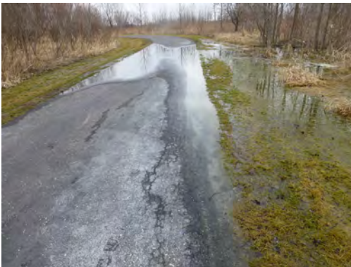
Seasonal pooling along trails were often associated with surface cracking.
