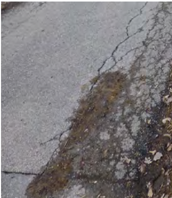
Alligator: Fatigue cracking associated with repeated traffic loading; exhibits as parallel longitudinal cracks that begin to interconnect
