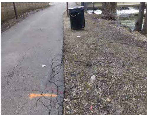
Edge conditions include cracking and disintegration of the trail surface.
