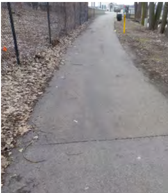
Transverse: Cracks that run perpendicular to roadway centerline; can be caused by shrinkage due to low temperatures or cracks in underlying layers
