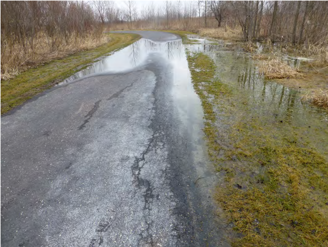
Inadequate drainage not only impacts the quality of the trail and reduces the lifespan of surface materials, it also creates an obstruction to trail use. Routine maintenance can help address these issues and provide for a more usable network.
