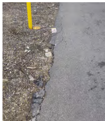
Edge Condition: Locations along pavement edge where pavement has broken away from pathway
