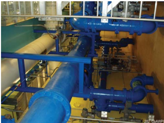
Filter Pipe Gallery with Filter-to-Waste at Oak Creek Water Plant
