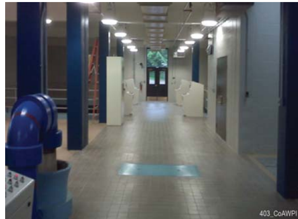
Filter to Waste Recycled to Filter Influent—Oak Creek Water Treatment Plant, WI
