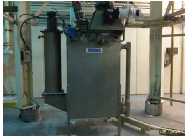
Water Treatment Facility Hydrated Lime Softening System
