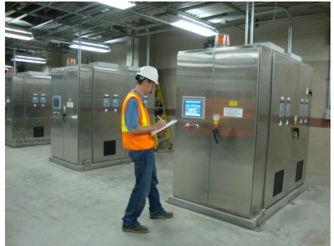
Todd Elliott, CH2M HILL engineer, operations assistance during Catskill Delaware Aqueduct UV system startup
