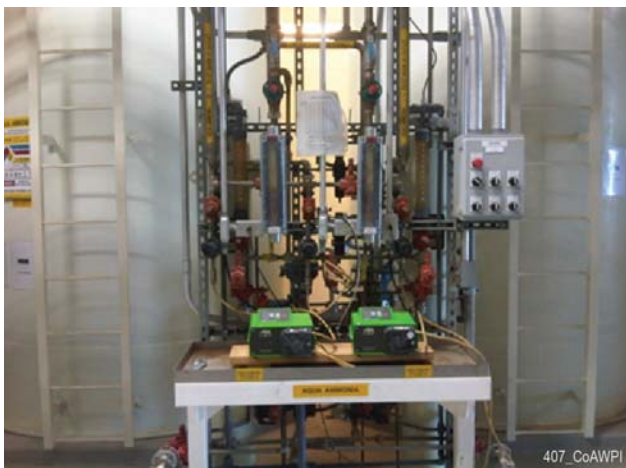
Water Treatment Facility Aqueous Ammonia System
