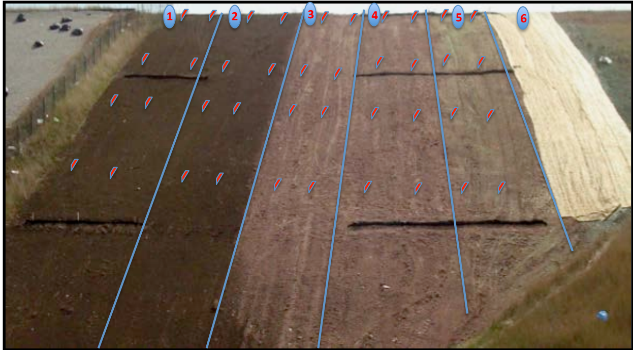
Figure 3.8: Finished erosion plot layout at the City of Appleton landfill site. Red dashes represent the placement of the wooden stakes used for the evaluation of erosion movement.
