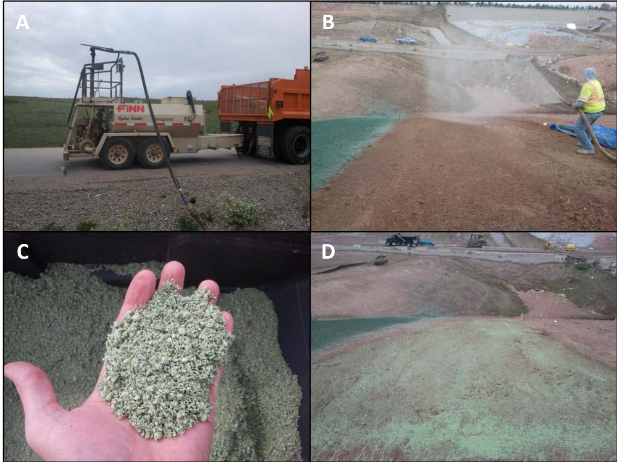
Figure 3.4: Preparation of plot five. A) Hydro seeder was used to apply the PAM-12 Plus product B) Application of product onto plot C) close up of dry PAM-12 Plus D) After final application of product
